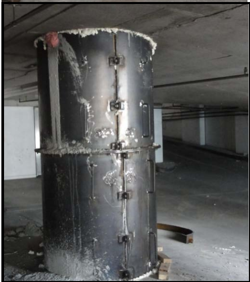
Damaged columns with completed encasement
